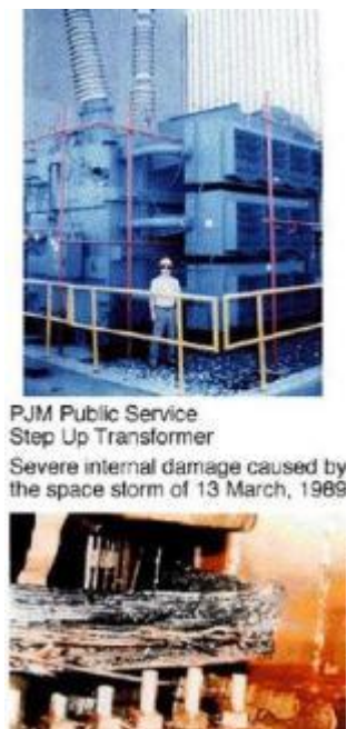
Figure 2. Burned Transformer in Hydro-Québec's power grid in 1989 [34]
